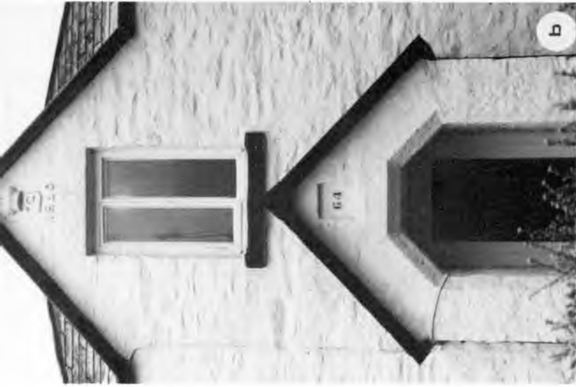
(b) Detail of Westbridge Cottages. Notice the rubble-stone wall (white-washed by present owner), granite porch and sills, and the ducal crest cast in concrete and set above the bedroom window.
